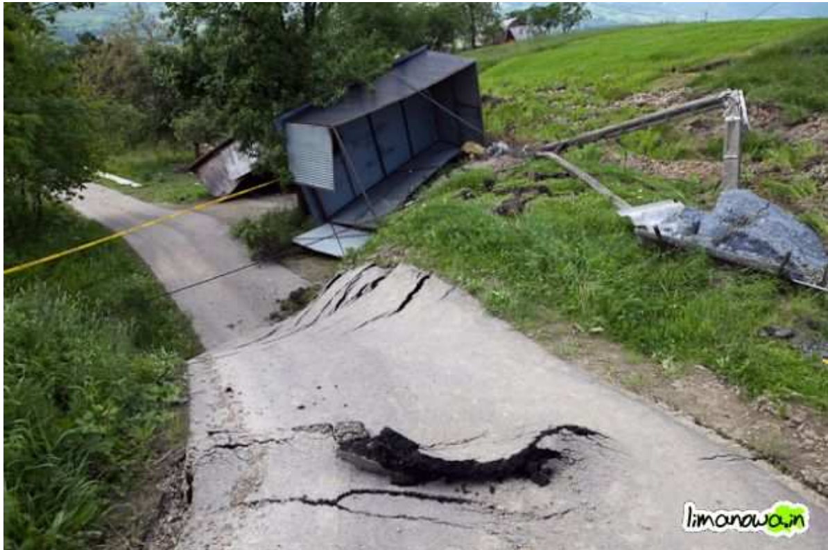
Fig. 7. A damaged road-landslides effect
