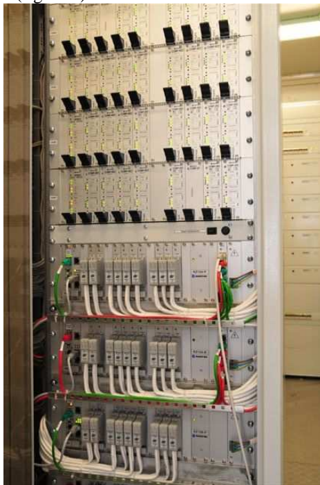
Fig.2. Block safe comparators and interlocking computers of MOR-3
